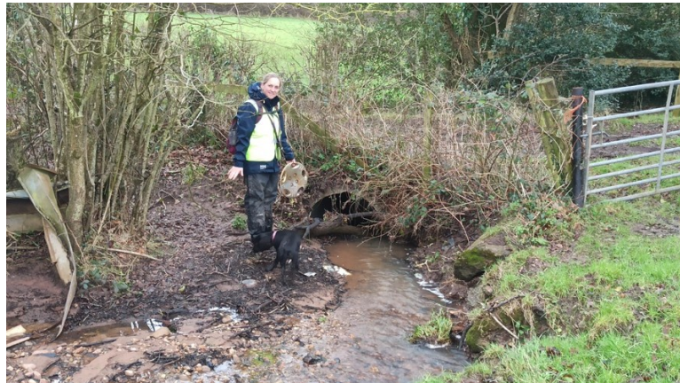
Single pipe can get blocked
