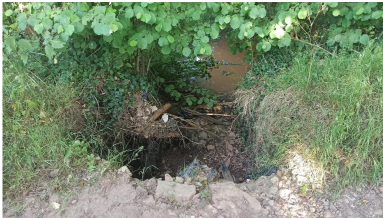
Erosion of track and river bank below track
