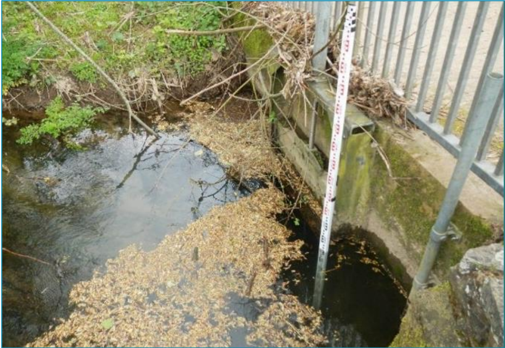
Photo 1: The Leat penstock- the proposed works will see the installation of 10mm aperture screening along with supporting walkways and guard rails.
