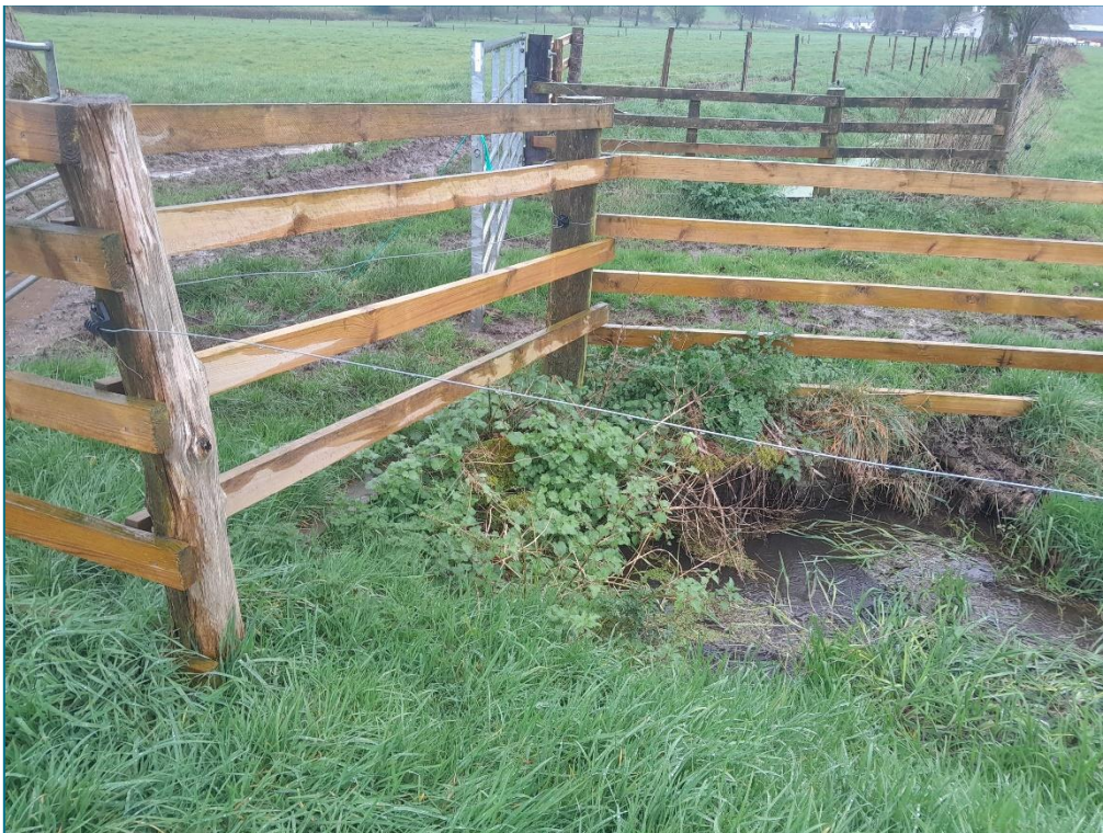
Photo 15: A view of culvert 2, this will need surveying and potentially improving ahead of construction.
