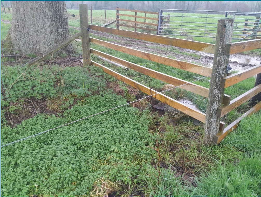
Photo 14: The Culvert 1 of 2 that will need to be improved ahead of site mobilisation.
