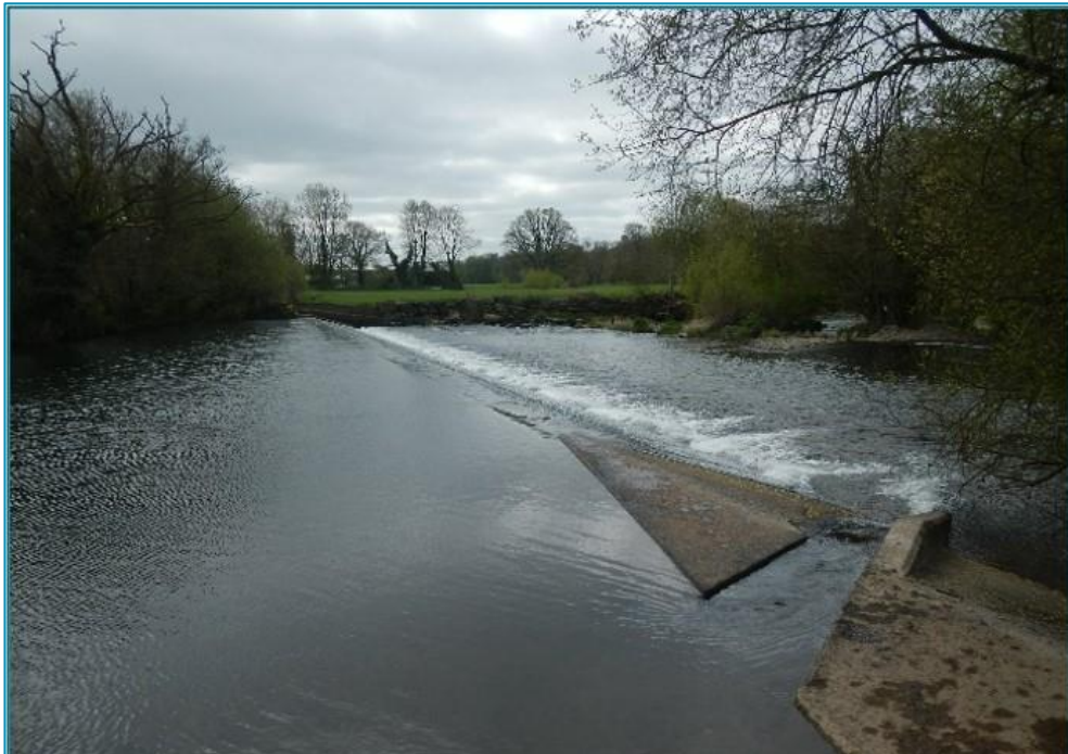
Photo 1: Looking downstream from the true right-hand bank of the weir, the silling basin is to be installed in the foreground of the photo. Also, in the foreground the current baulk- pass that is to be removed and profiled back to the weir glacis.
