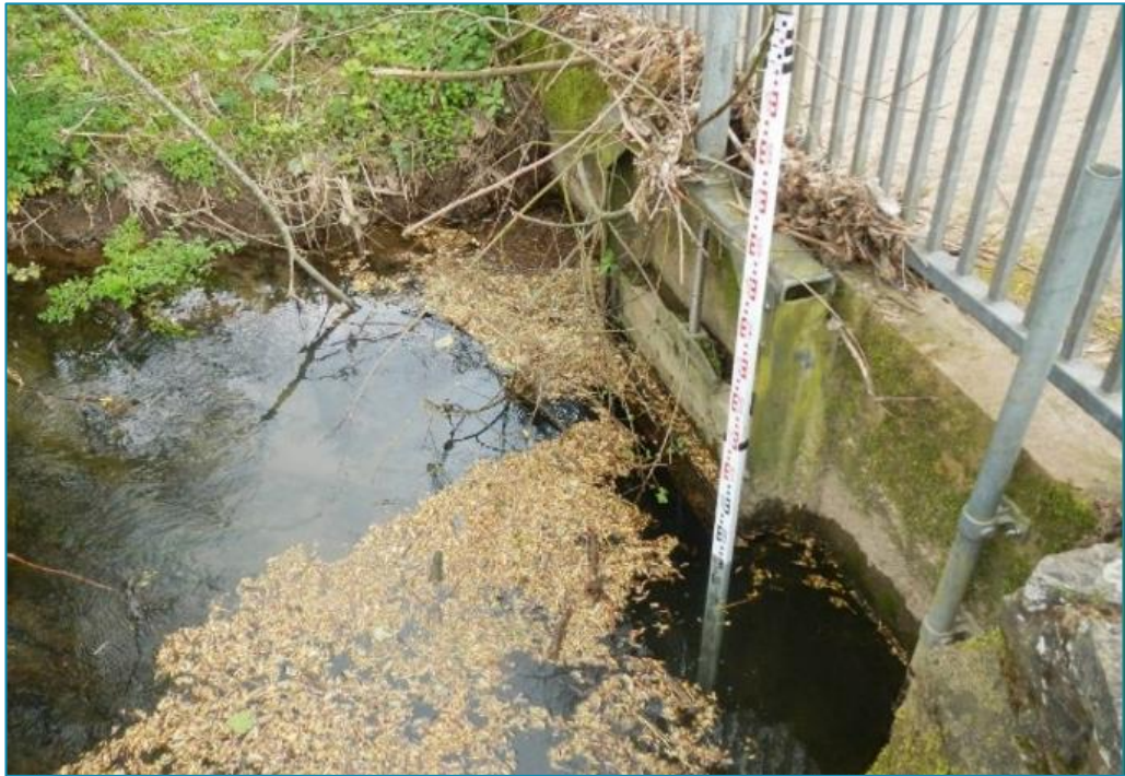
Photo 4: The Leat penstock- the proposed works will see the installation of 10mm aperture screening along with supporting walkways and guard rails.
