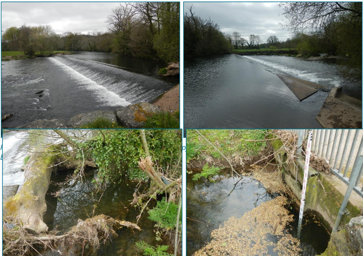
Plate 4: Details of channel leading to leat inlet and channel immediately upstream of leat inlet. Abundant cover may attract eels towards the leat inlet. Location at the downstream end may attract downstream migrating fish.
