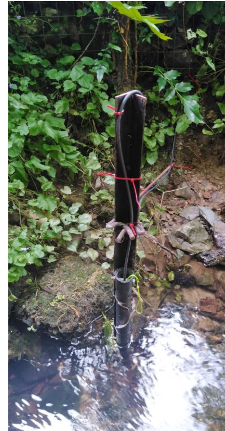
Fig. 4 The AT200 sonde in its casing. It is installed so it sits upright inside the pipe to avoid it getting damaged or clogged with debris and sediment.
